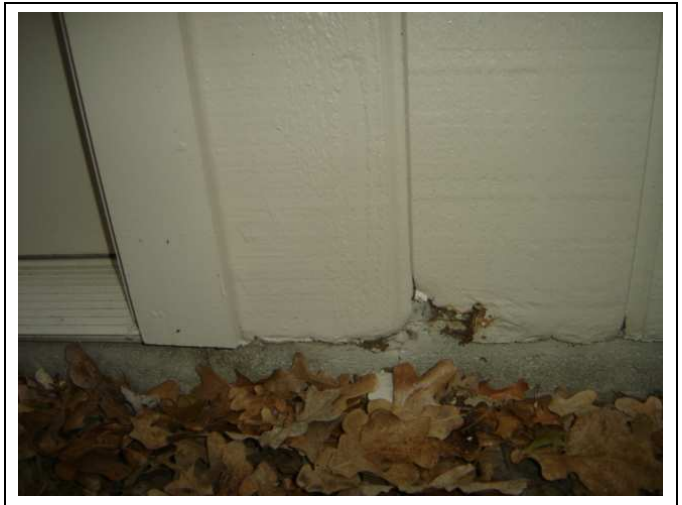
Wood rot to siding, rear of house
