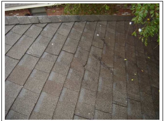
Tree limb damaged shingles
