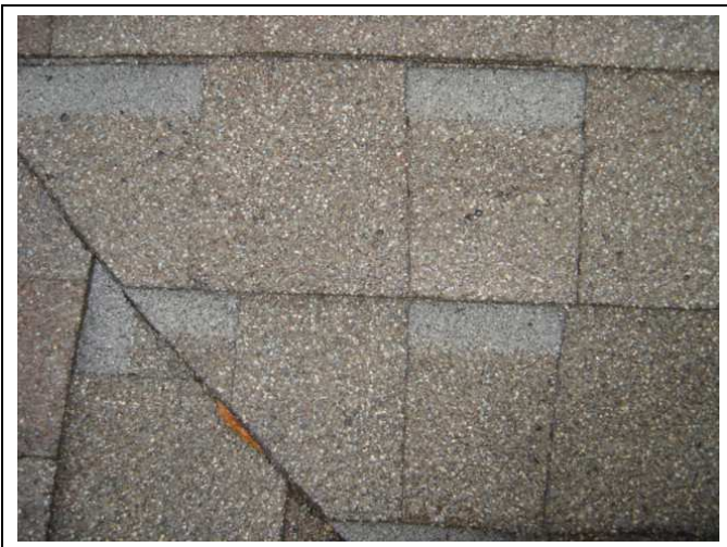
Blistered shingles on roof
