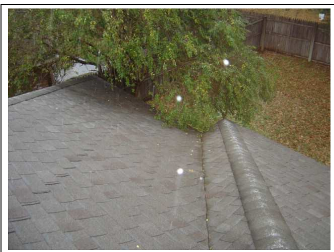
Tree limbs in contact with the roof
