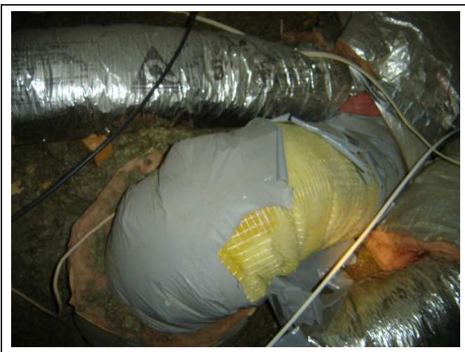
Deteriorated ductwork, attic
