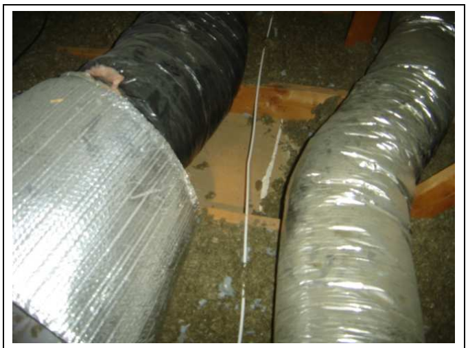
Area of attic not insulated
