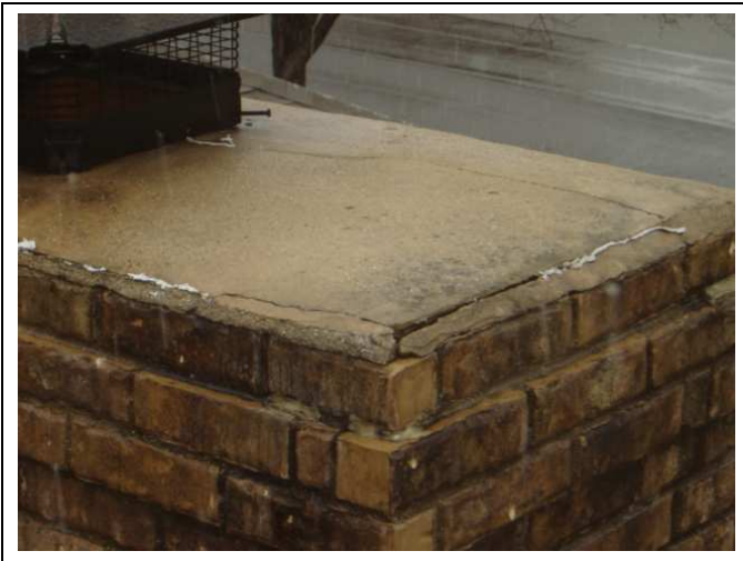
Cracks in chimney mortar cap, roof
